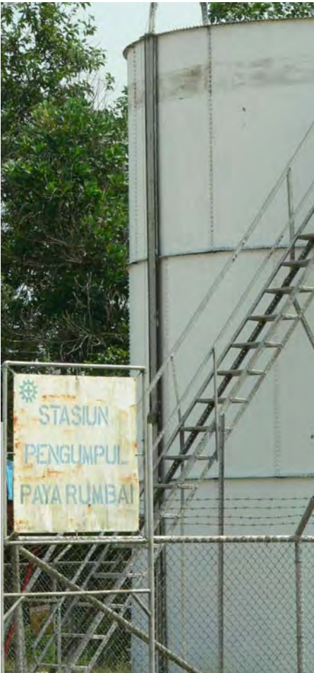
Palm oil storage tank, Riau (photo: DTE)
